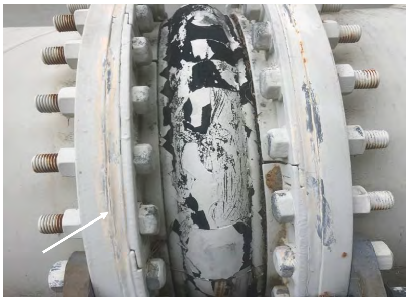
Photograph 6 – Korblex – 2 MG reservoir – West wall at 2' O.D. Flange – Paint (white) reported to contain lead.
