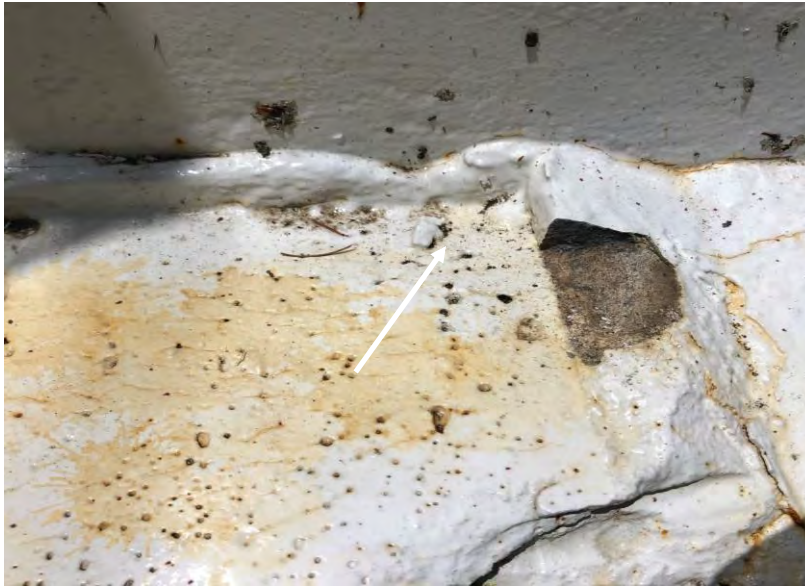
Photograph 9 – Korblex – 1 MG reservoir – Paint (white) at pad and tank intersection reported nondetect for asbestos and reported to contain lead. -
