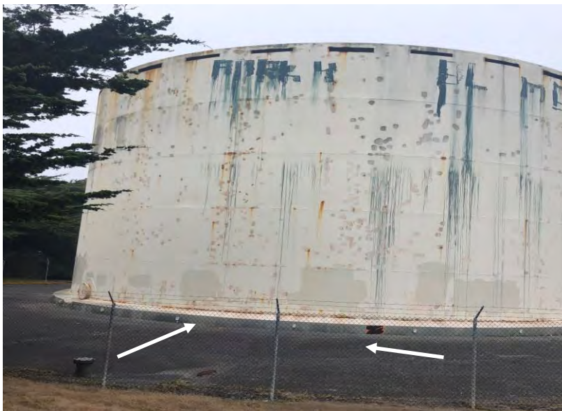
Photograph 12 – Samoa – 1MG reservoir – Asphalt (black) and concrete pad (grey) reported to be nondetect for asbestos.
