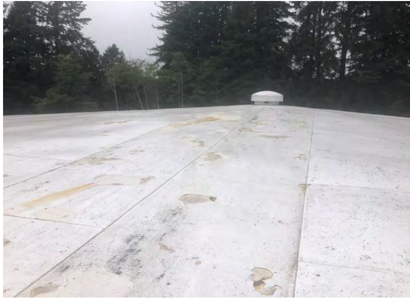
Photograph 5 – Korblex – 2 MG reservoir, roof paint and surfacing coating reported to be nondetect for asbestos and lead.
