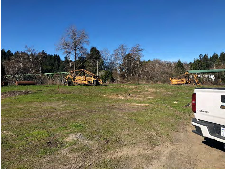
Figure D11. Facing northwest showing the staging/laydown area on the east side of the river.
