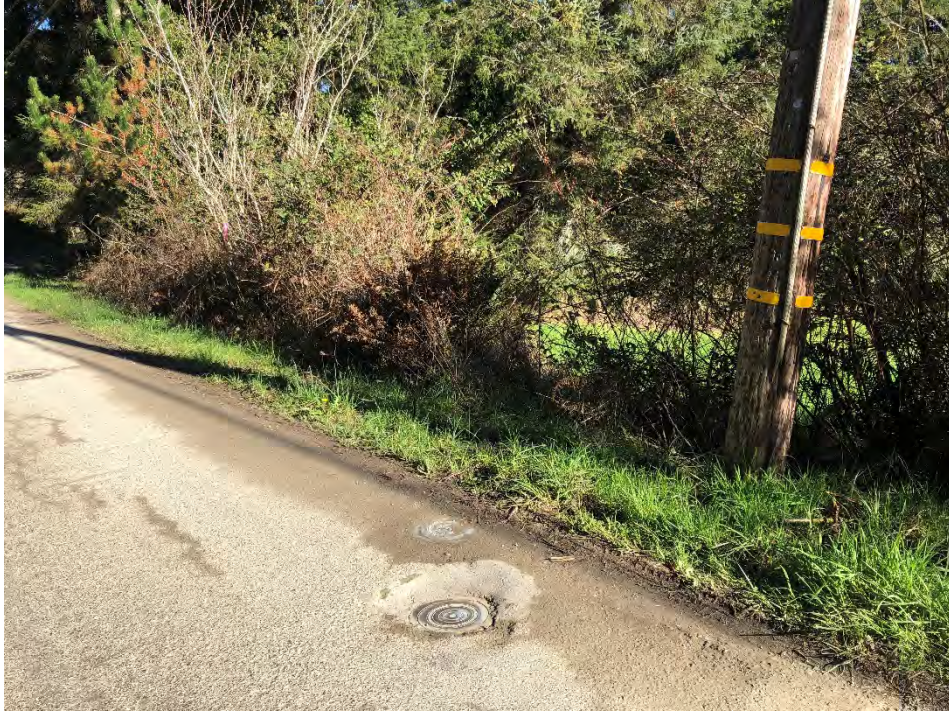
Figure D9. Facing north on Warren Creek Road showing the existing valve boxes at the location of the modification of the existing river crossing.
