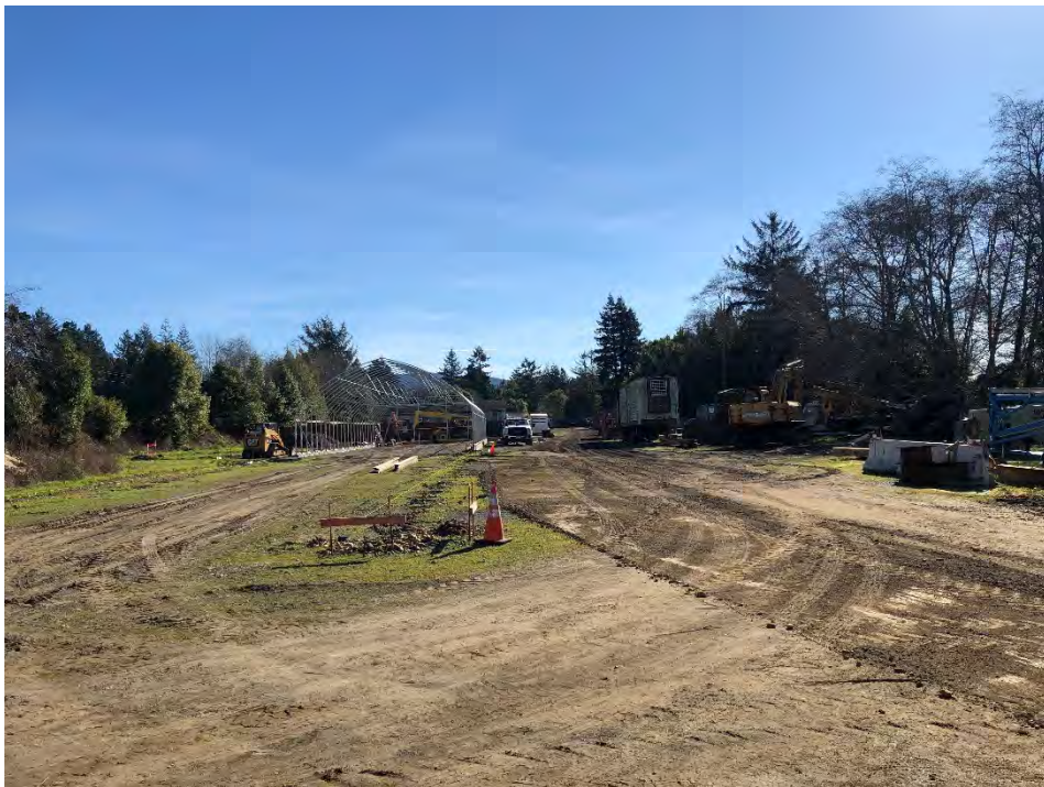
Figure D10. Facing southeast from the staging/laydown area on the east side of the river showing the construction access road towards Glendale Road.
