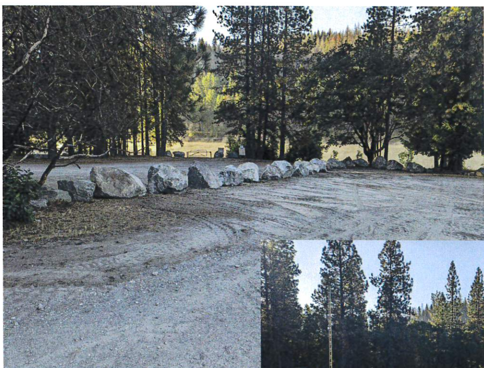
Boulders in place at Old Ruth to prevent unauthorized lake access (final placement)
