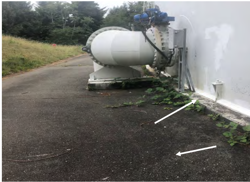
Photograph 7 – Korblex – 2 MG reservoir – Asphalt (black) and concrete pad (grey) reported to be nondetect for asbestos
