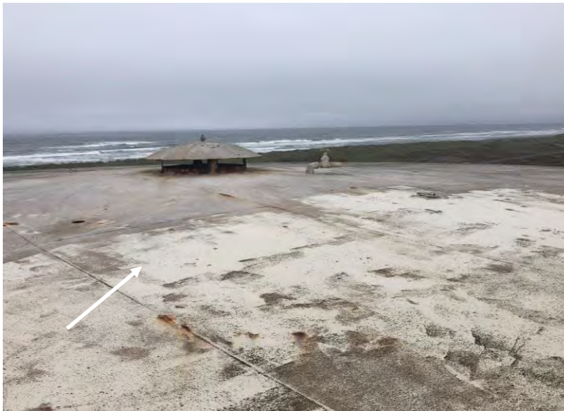
Photograph 10 – Samoa – 1 MG reservoir – Roof exterior paint (white) reported to be nondetect for asbestos and lead.
