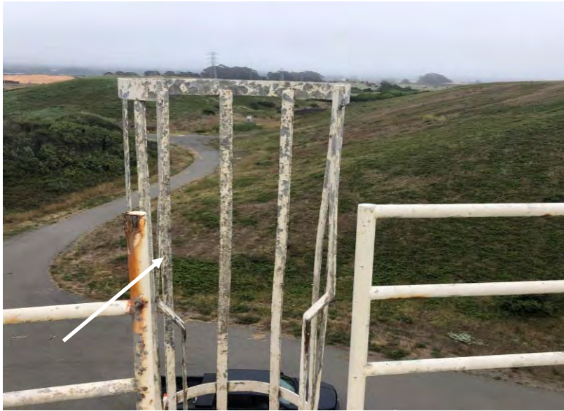
Photograph 11 – Samoa – 1 MG reservoir – Paint (white) located at roof east handrail reported to contain lead. -
