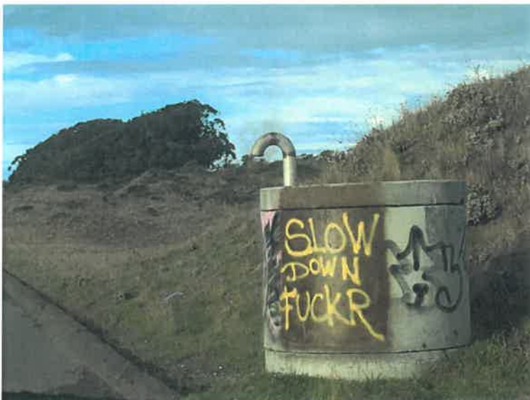
Above: one of the concrete vaults bore this message for many months.
