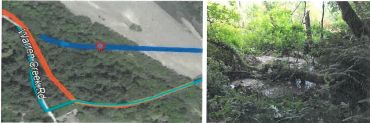
Figure 12 – Location of surface return of drilling fluid (red) with corresponding bit position (blue arrow). Pool of fluid accumulated at the base of the steep canyon (right photo).
