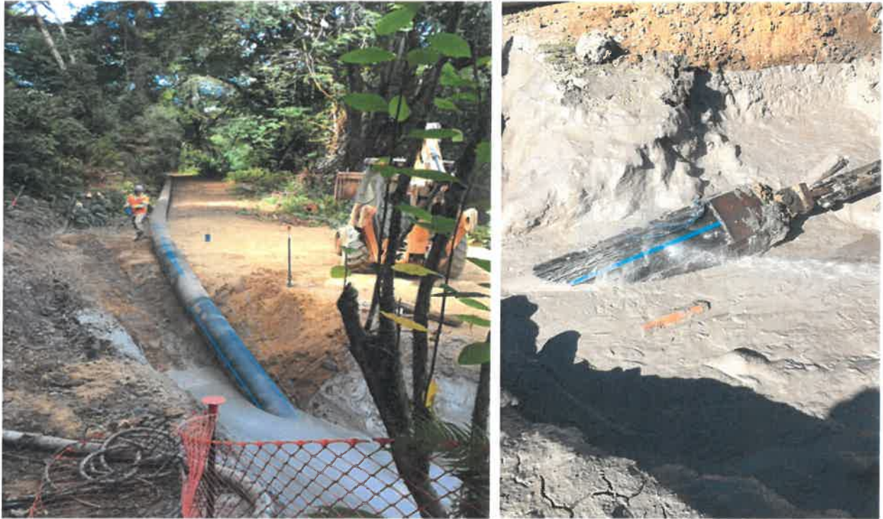
Figure 14 – Carrier pipe transitioning from abandoned railroad grade into exit pit (left); pull head arriving at the entry pit at the completion of pullback (right).
