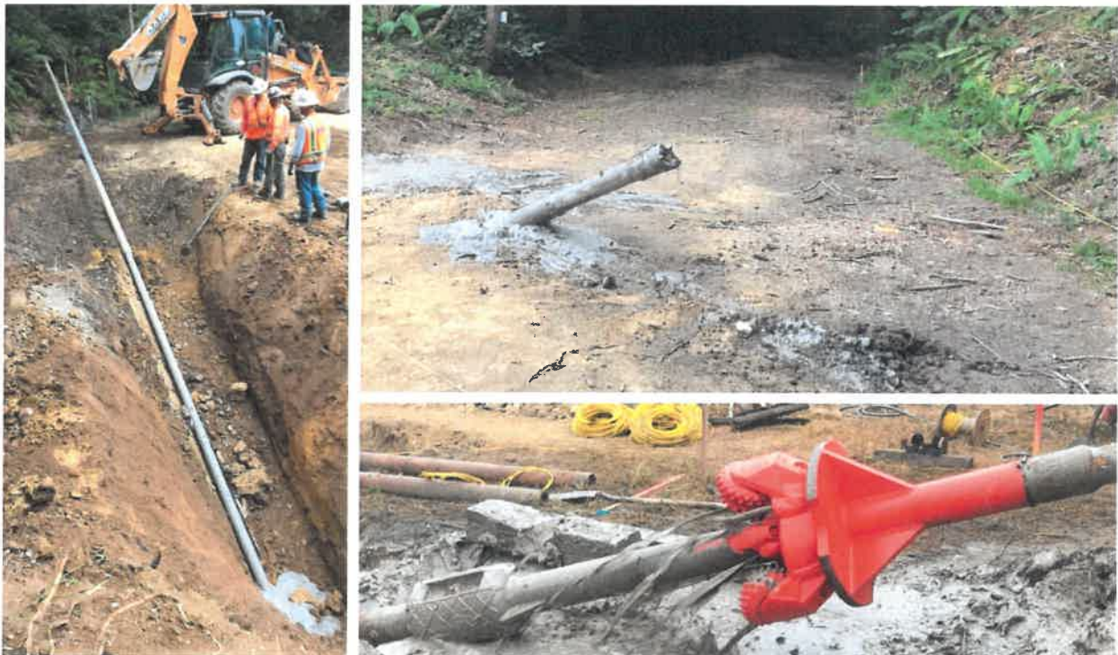
Figure 13 – Exit location of the pilot bore (upper right); deep pit excavated at the exit location to allow for transition of the carrier pipe into the bore (left); and the 27" reamer connected at the entry pit (lower right).
