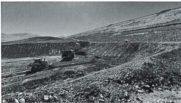
Heavy machinery excavates slope wash from the base of B.F. Sisk Dam
