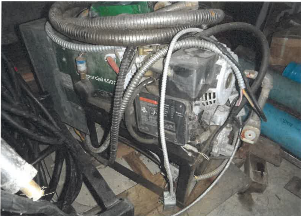
Commercial 4500 propane generator (ran when removed from service)
