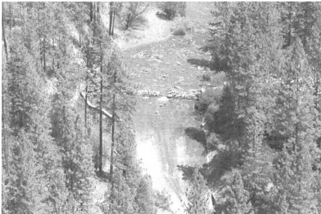
The spillway at Misselbeck Dam west of Redding has been deemed unsafe by state officials. (Photo: Igo Ono Community Services District)
