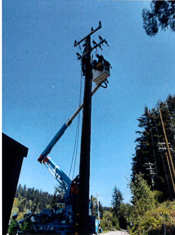
PG&E Hookup to 12kV
