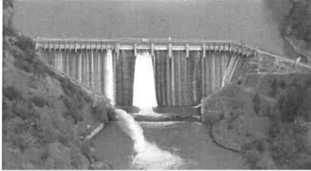
Scott Dam at Lake Pillsbury — a key component of the Potter Valley Project. Photo: PG&E.
